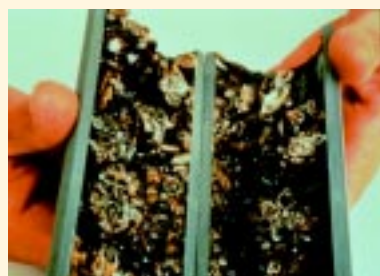
Zebra Mussel populations can completely restrict flows in intake pipes. Department of the Interior, United States Geological Survey, Photo by Don Schloesser
